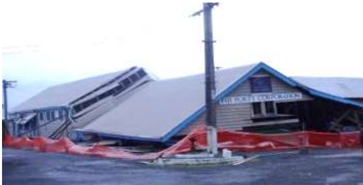
Figure 28 Damaged Fiji Ports Building
