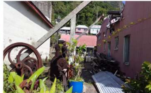
Retail Store with Top floor blown. Concrete brace remains
