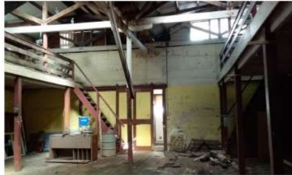
Public Gym - Damages from Cyclone
