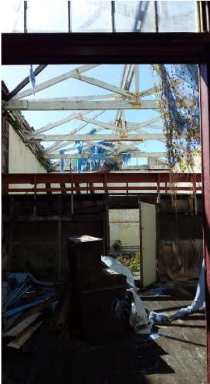
Squash court roof damaged - Lack of funding stalls repair works causing damage everyday
