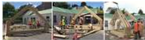
Figure 4 1:1 scale prototype of six portal frames on-site at the Institutes workshop . This prototype was vital in the progression of the project.
