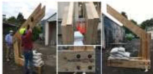
Figure 3 1:1 Detail Prototype: This was used to test for tolerances, check connection details, gauge material aesthetics before material was ordered.
